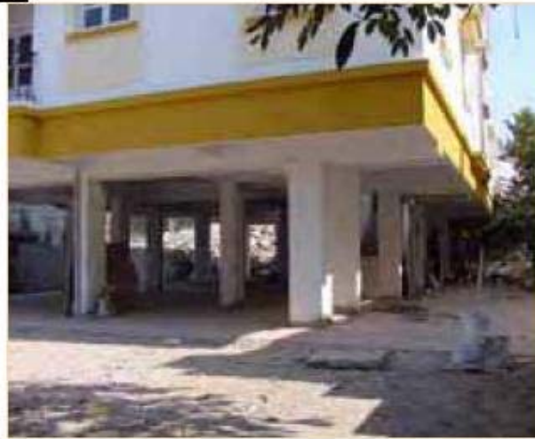
Figure 24. Typical building with a soft ground story in India (source: EERI 2001).
