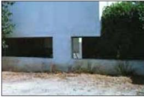
Figure 17. A building with short columns at the basement level in Cyprus (source: Levitch 2002).
