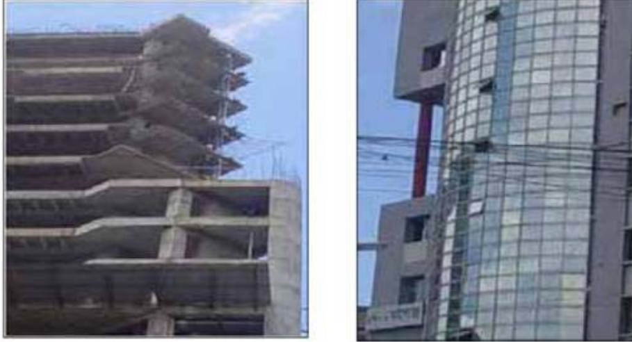
Figure 10. Examples of vertical irregularities (from Bangladesh) that can induce undesirable torsional effects (source: M. A. Noor).
