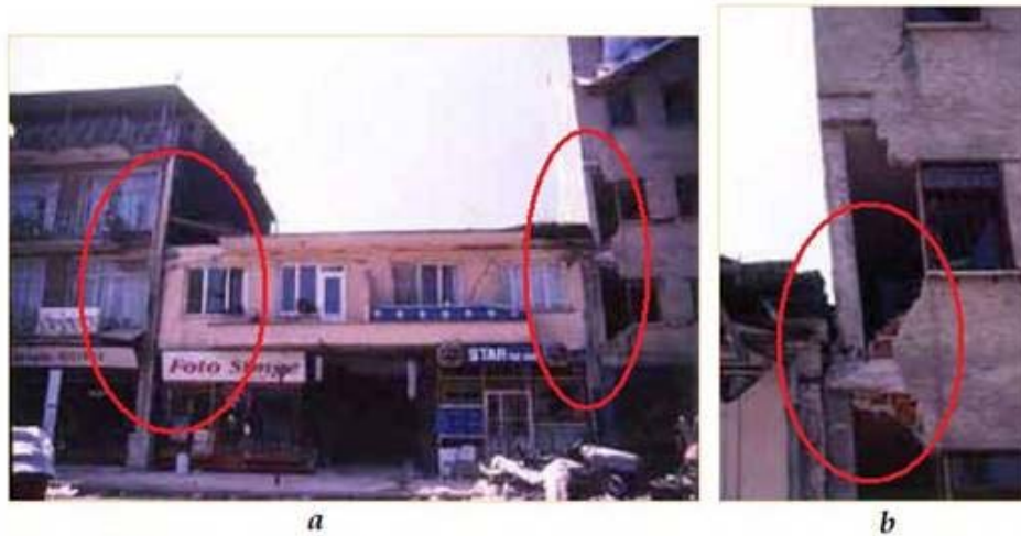
Figure 23. (a) Pounding between a six-story building and a two-story building in Golcuk, Turkey causing damage in the column of the six-story building, (b) Detail of pounding damage in a six-story building shown in figure (a). (source: Gulkan et al. 2002).
