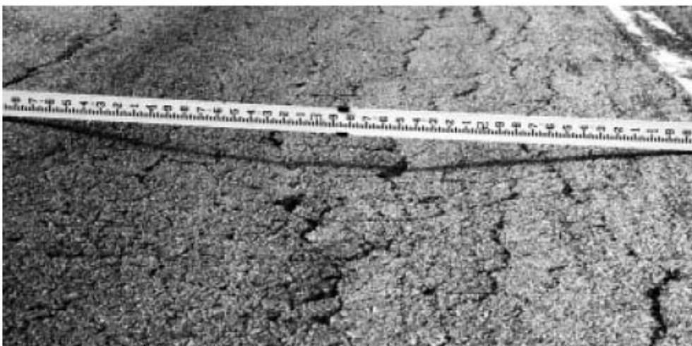
◀ Severe rutting caused by poor base or subgrade.
